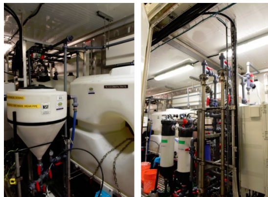
Figure 3-2 Pretreatment Lime Dosing System (left) and Filter System (right)
