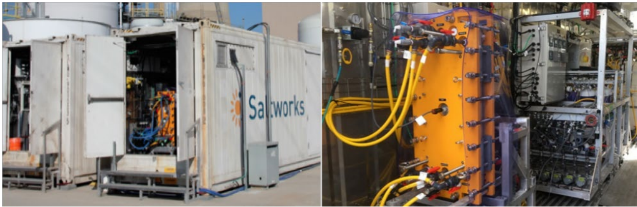
Figure 3-1 Flex EDR Selective with Pretreatment Pilot Plants (left) and Flex EDR Selective Stack and Control System (right)
