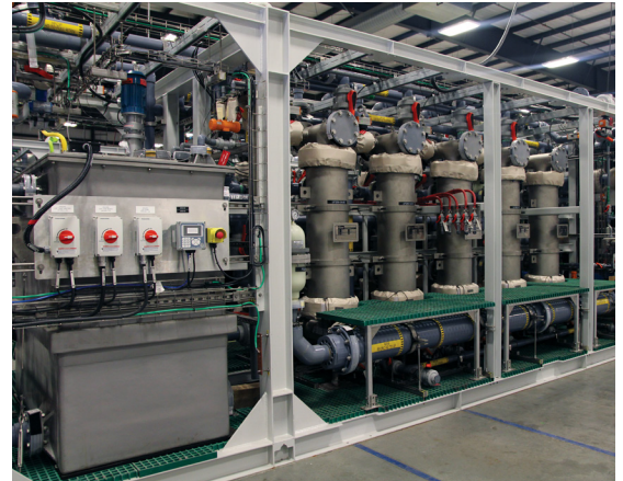
A section of an XtremeUF plant
